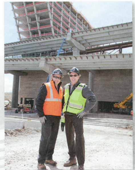
Jon and Rick Kinning on-site at the Westin hotel project at the Denver International Airport.
